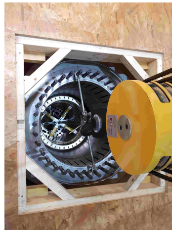
FIG. 111. Installation of the external Bitter coil inside the warm bore of 814 mm diameter, seen from the mezzanine covering the upper part of the hybrid magnet cryostat.
