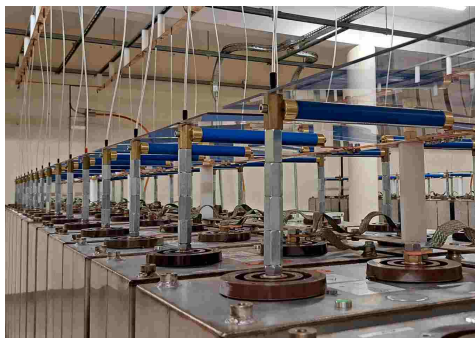
FIG. 120. Photo of the 1\text{ M}\Omega resistors, the blue cylinders, installed on the capacitors for the automatic discharge. The fuses are the small vertical tubes above the resistors.
