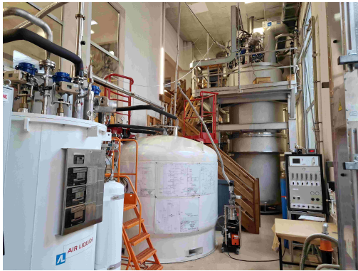
FIG. 112. Overview of the core part of the cryogenic utilities with on left side the He liquefier cold box connected to the intermediate dewar of 4500 l providing LHe to the cryogenic satellite producing the pressurized superfluid He to cool down the superconducting magnet.
