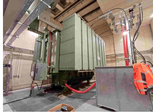
FIG. 102. Installation of the new transformer in its building after assembly of the two side heat exchangers. On the right, one distinguishes the departure of the 15 KV orange lines connected on the other side to the HTA Cells located in the LNCMI building.
